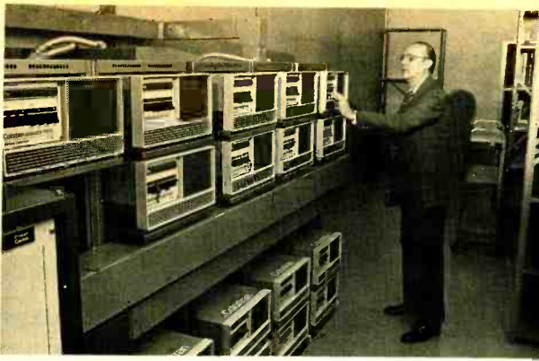
Ed Steeb checks out one of seventeen Colortran Dimmer Packs which control 102 lights, and are balanced for phase.
