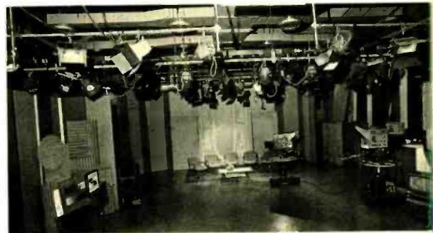
Sets can be lit in any of a combination of ways, using a wide variety of quartz-iodine lights.
