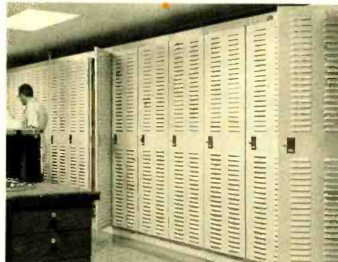
Back side of equipment racks form one wall of maintenance shop.
