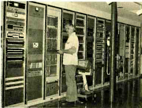
Equipment racks along rear wall of Master Control room, Assistant Chief Engineer, Leo R. Huber, is shown taking measurements.
